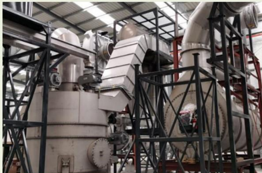
Torrefaction line: 2,70 m swirl reactor incl. 500 kWth heater
